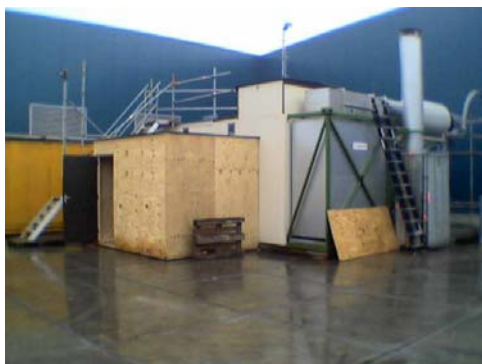
Left: The ORC power plant in use at the test facility of Tri-O-Gen in Goor, Holland (the power plant is assembled to a standard container, which makes transport easy). In this cite the plant is run by burning natural gas, but later the plant will be transported to its final cite, where fuel will be biogas.
