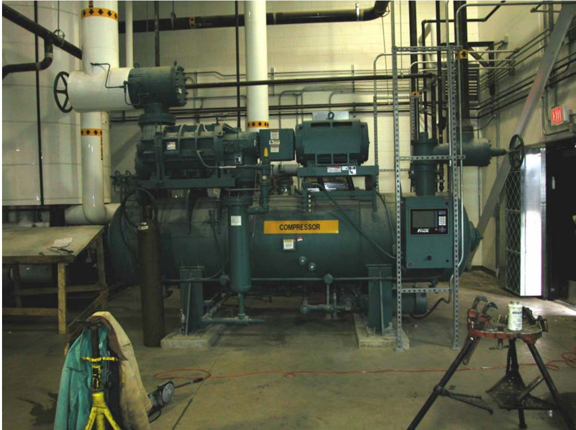
Figure 3 – Low Temperature Booster Compressor
