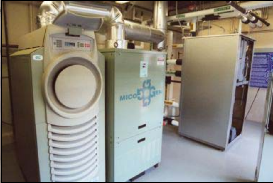
Figure 2 Microturbine, Heat Recovery Heat Exchanger and Absorption Chiller
