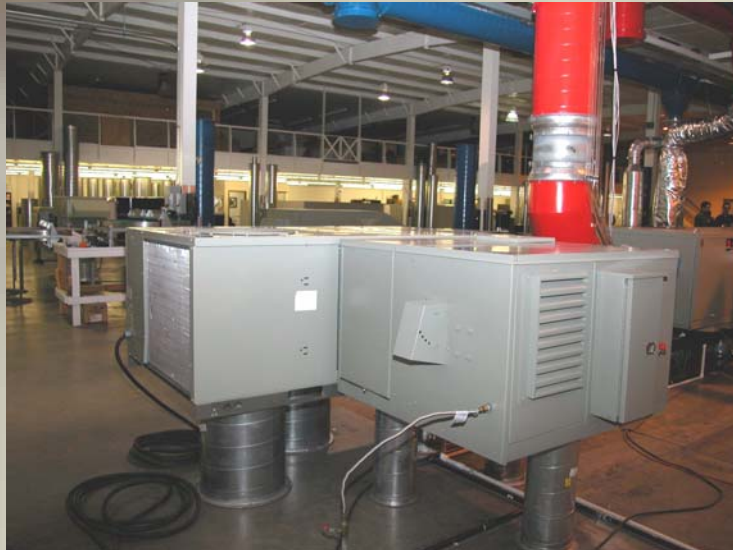
Figure 2 – 10 RT Rooftop with prototype ADM (foreground) on Test
