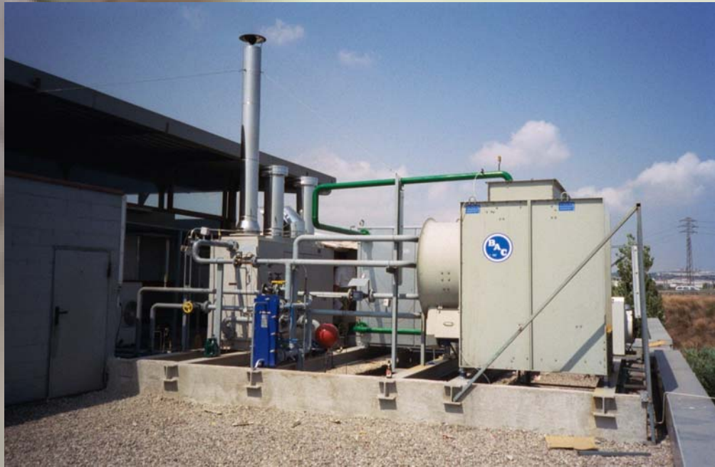
Figure 2 - Bowman 80 kW Hot Water CHP with Absorption Chiller and Cooling Tower
