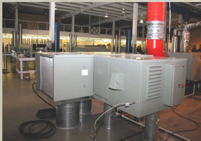
Figure 2 – 10 RT Rooftop with prototype ADM (foreground)
