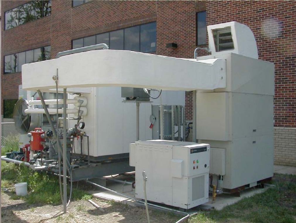
Figure 3 - 60 kW Microturbine, Broad nominal 50 RT Absorption Chiller with Cooling Tower
